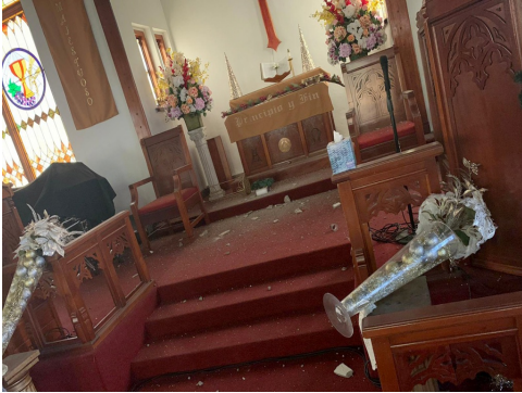
The Methodist Church of the Resurrection in Ponce, Puerto Rico, suffered extensive damage in a series of earthquakes that have rattled the country since December 28 th . (Photo courtesy of the Methodist Church of Puerto Rico.)
